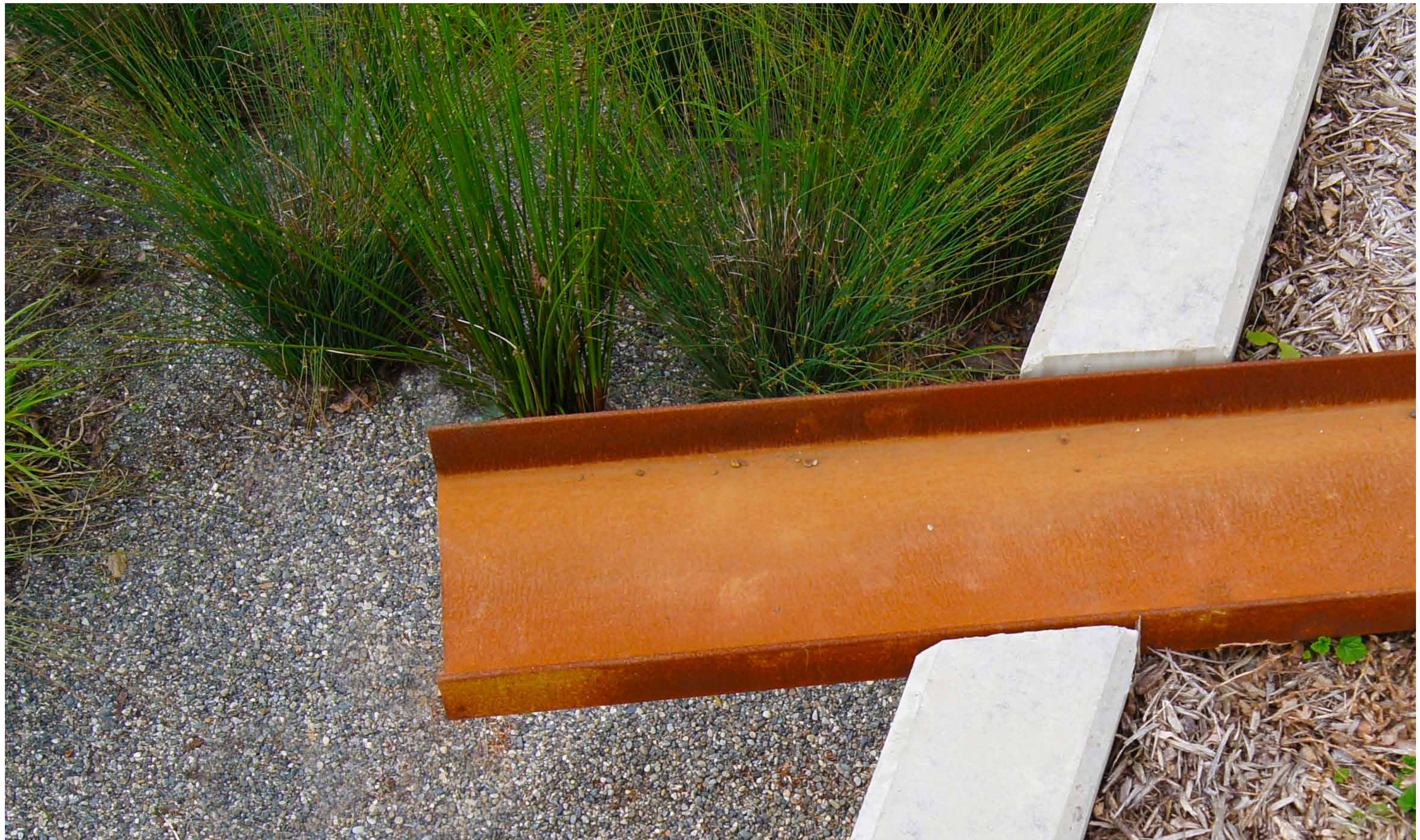
Bio-retention: Detail view of a channel surface runnel that directs water to the bio-retention planter.
