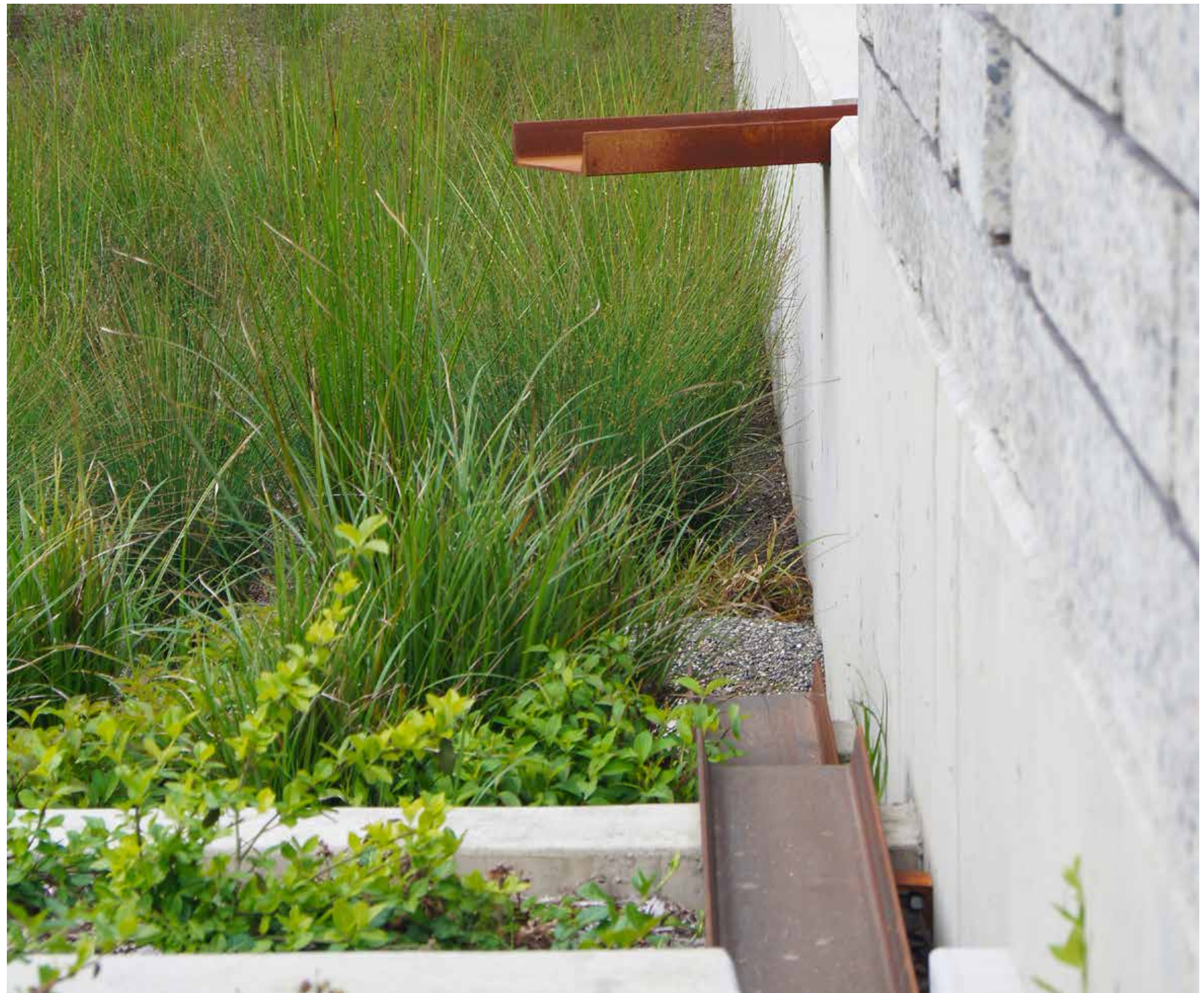
Recycle Water: Salvaged building materials direct water from the reconfigured roof, and previously untreated parking areas, via at-grade runnels to the bio-retention planter that was once the loading dock.
