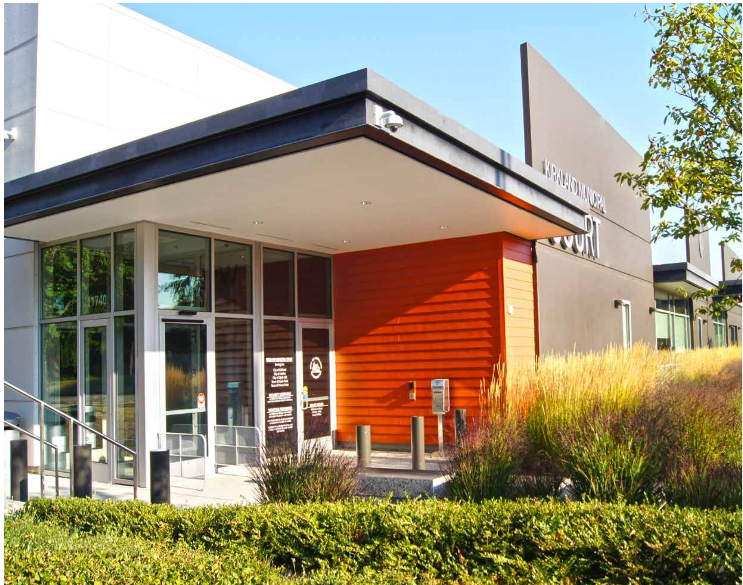
Remove Panels: Existing tilt-up precast walls were removed in strategic locations to allow for new entries and windows to soften the new interior spaces.
