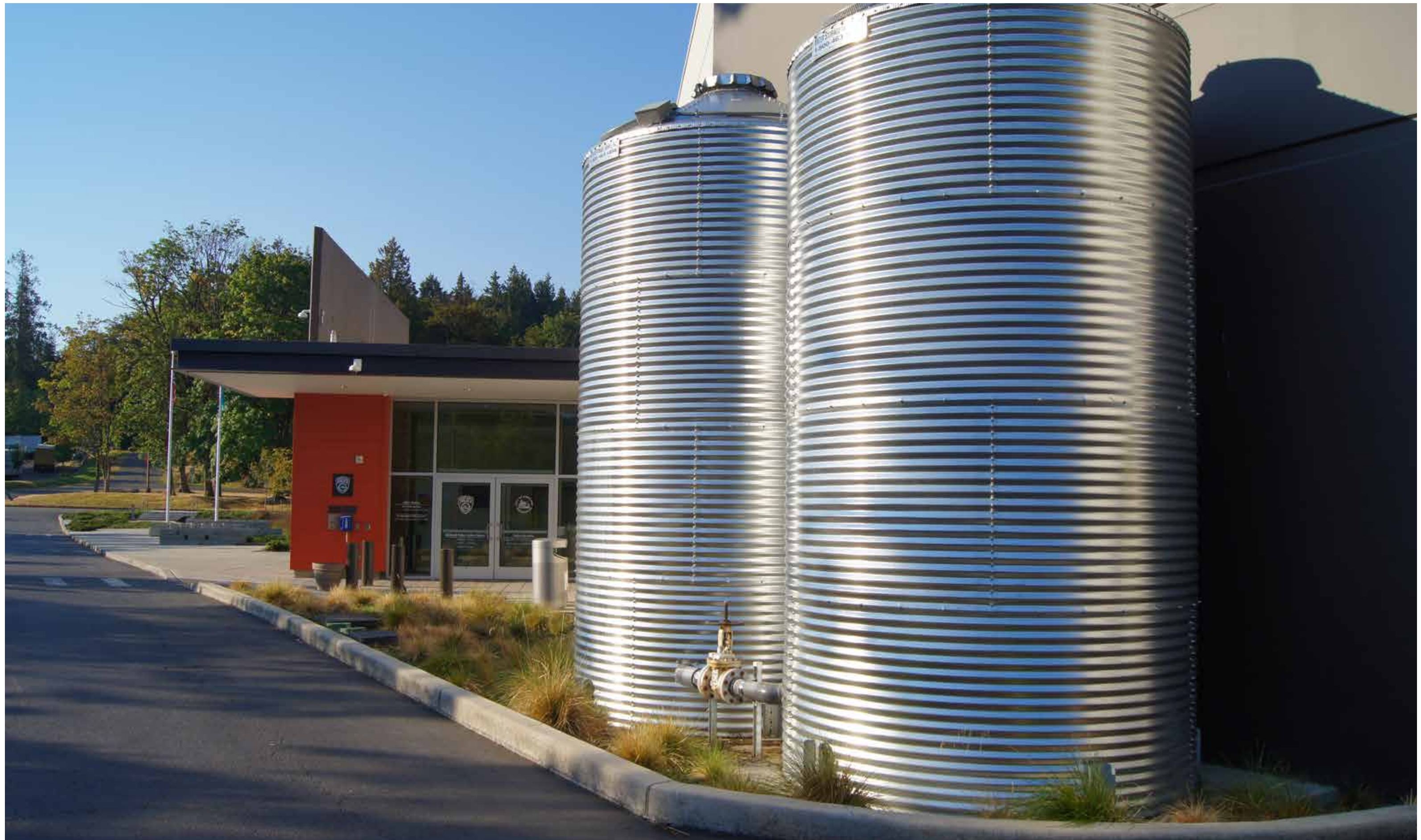
Rainwater Cisterns: Rainwater from the roof is captured in two corrugated metal cisterns, conveying the city's desire to exhibit sustainable strategies to the public. Captured rainwater provides 100% of the irrigation needs for the new landscape.
